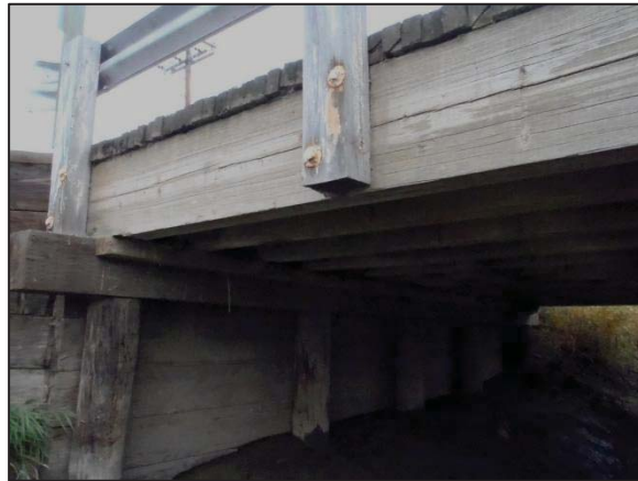
Figure 4 Untreated girder in bridge 724
