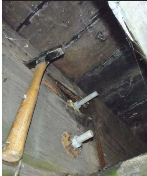
Figure 5 Decay in G14 of bridge 1302
