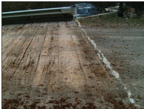
Figure 11 Wheel path depressions in timber deck on Shovel Creek Bridge
