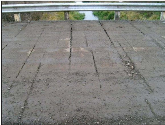
Figure 3 Deck cracks in bridge 724
