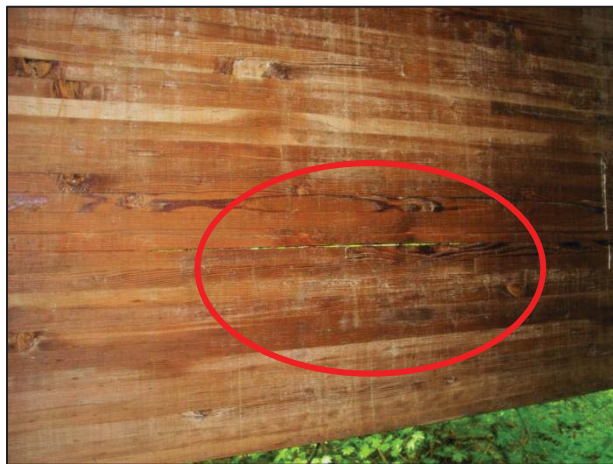
Figure 9 Horizontal shear crack in Griffin Creek bridge
